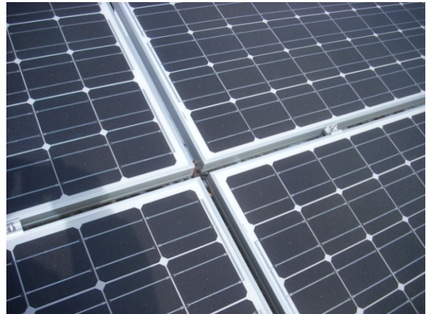
Detail of solar panels
