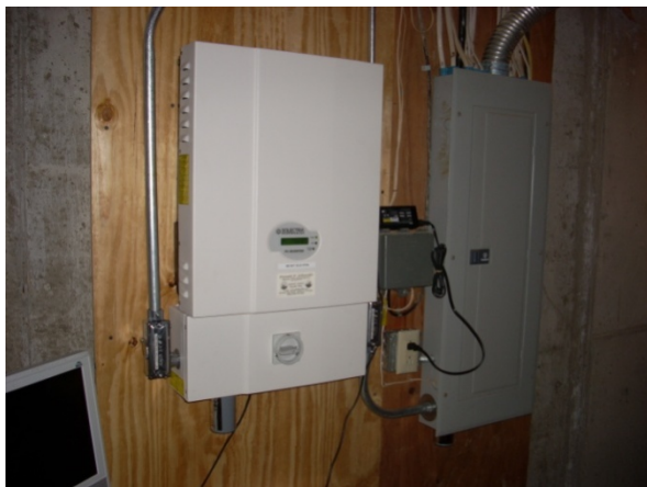
5000 watt inverter mounted by panel in basement
